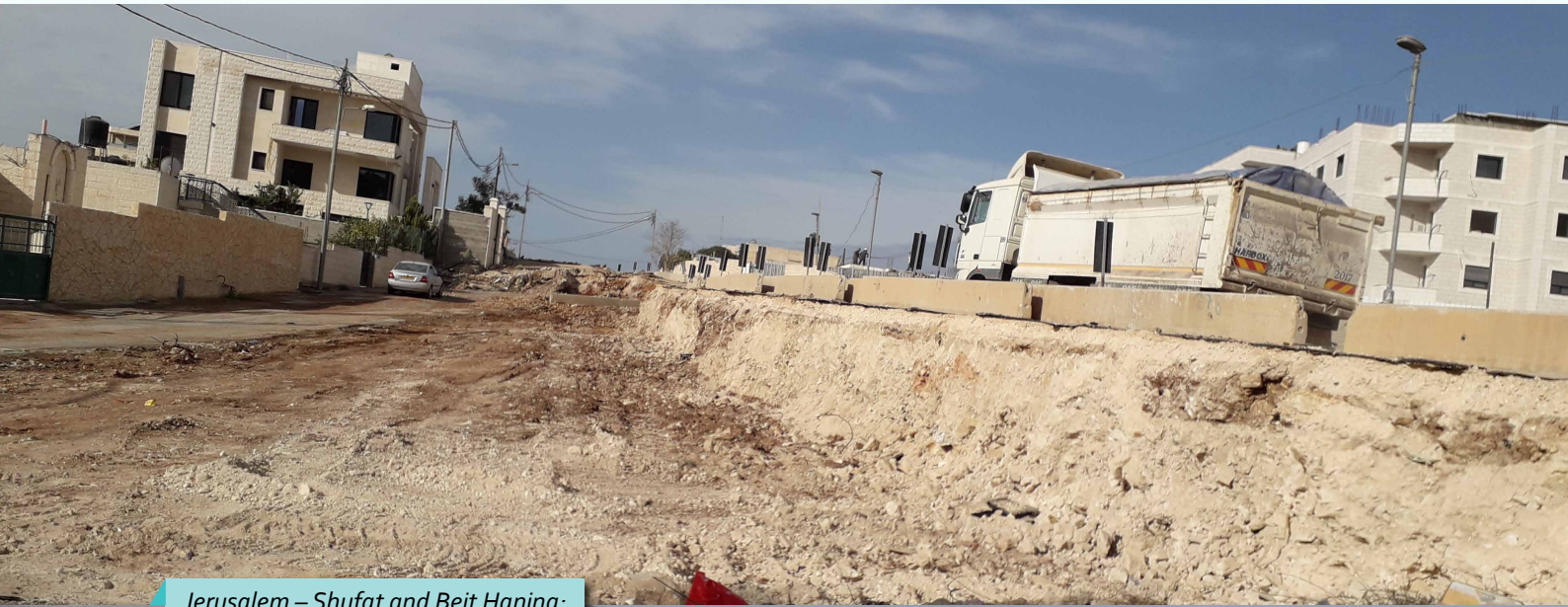
Jerusalem – Shufat and Beit Hanina: Opening the fourth segment of bypass road no. 21 – January 2018
